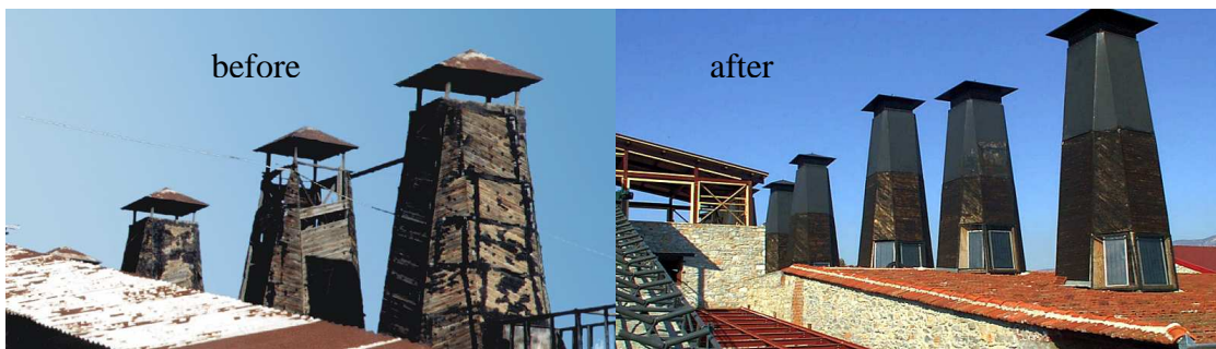
Figure 2. Chimneys of the old drying rooms before and after the rehabilitation. The rehabilitated chimneys function as solar chimneys for natural ventilation. The way the solar water heating collects were incorporated in the base of the chimneys, is also shown.
